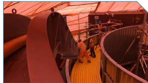
Nexans Makes Final Cable Delivery to Canada's Strait of Belle Isle Subsea HVDC Power Link
