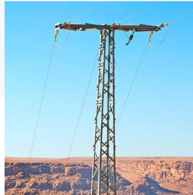
MoU FOR A MEDIUM VOLTAGE GREENFIELD IN MOROCCO
